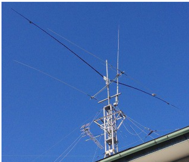
Three antennas on the roof tower.
