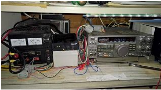
Part of the GW3YTC Remote Controlled Station (G4ZLP Digimaster Pro 3 CAT Controller & Interface Box Centre)
